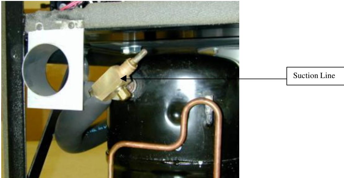
Figure #3 Suction line orientation
